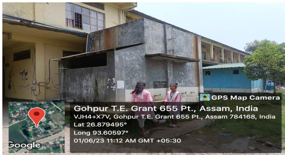
Water Tank and Storage Facility
